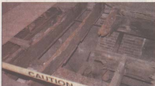
This hole is the most obvious example of what's going to take money to fix in the Carnegie Library. The hole was the result of a leaky roof that pooled water in one spot on the top floor for years. The roof has since been replaced but the leak damage remains.
